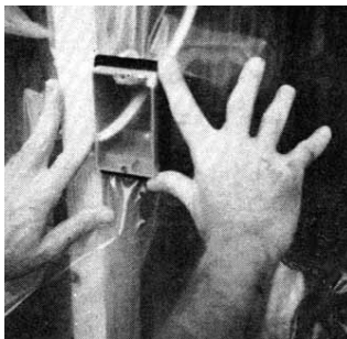
Figure 1. R&S boxes provide a relatively easy and inexpensive seal. Romex wiring enters the box through a neoprene patch. A plastic snap-on ring seals the box to the poly, which is slit to allow access to the wiring.
