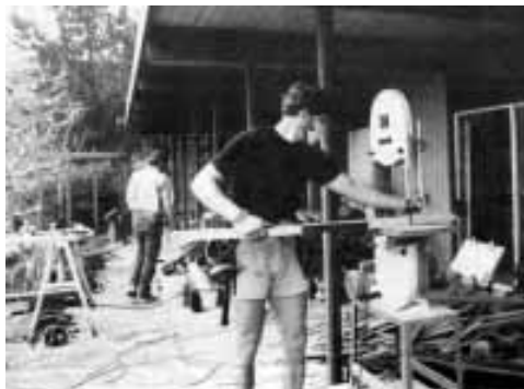
Figure 3. Building curved decks requires a lot of equipment, including a bandsaw for cutting caps and rails, and a planer for reducing the thickness of the fascia. The author hauls tools and hardware to jobs in a covered trailer, and then rolls them into place on sleds with castors.
