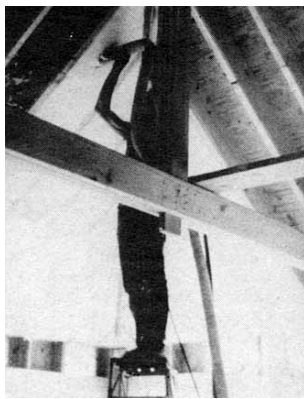
Figure 1. Using Ark-Seal's "Blow-In-Blanket" system, a contractor pumps loose-fill fiberglass, with a little water and adhesive, into a rafter cavity covered with nylon netting. Here, the cavity is blown full with no air space above the insulation, creating an unvented "hot roof."
