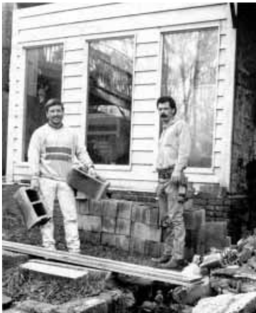
Crew members Jim Kearney, at left, and Tim Joyce at the site of an Atlanta addition.
