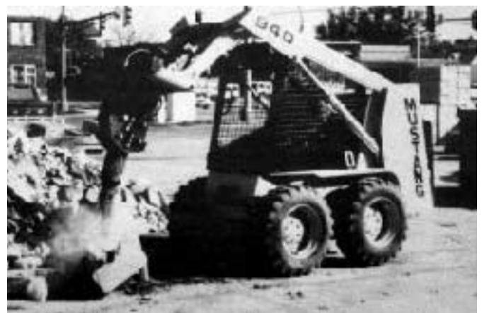
If you need to break up a large slab and have the room, consider renting a hydraulic breaker that mounts on the front of a skid steer.
