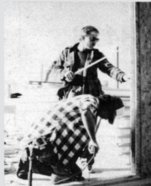
Wiring. Most wall panels come with predrilled chases for electrical wiring. Before setting a panel in place, drill a 1-inch hole through the subfloor to align with the vertical chase in the panel. Fishing wire is then fairly simple.
