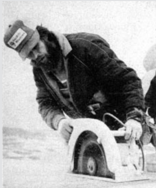
Cutting. You'll need an oversized saw to cut any panel. For those too thick for the saw, use a small chainsaw so you don't have to flip every panel for a second cut.
