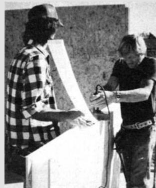
Notching. To let in nailers for the window or door frame, you'll have to notch the foam. This is easiest using the hot-wire tool shown here, supplied by most manufacturers.
