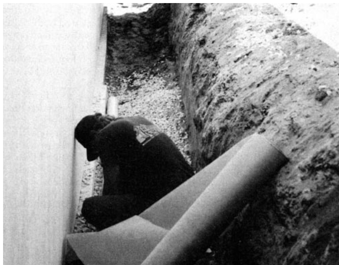
Figure 2. The 3-foot bucket on the author's excavator creates a trench that's easy to work in.
