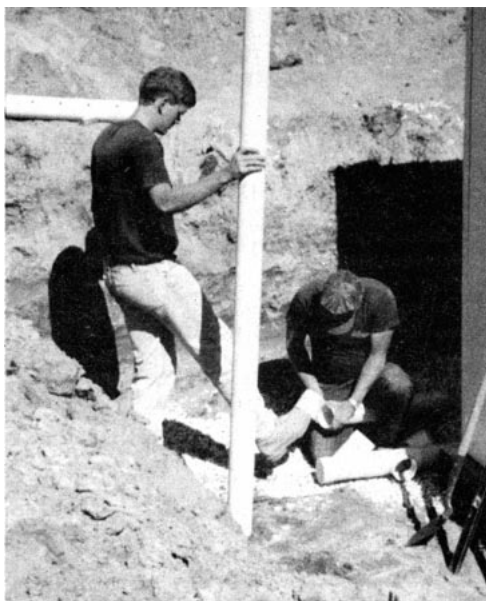
Figure 5. The author always includes cleanouts at every corner of the drainage system for periodically flushing the pipe. At left, he fits a wye for running the flush tube up to grade.
