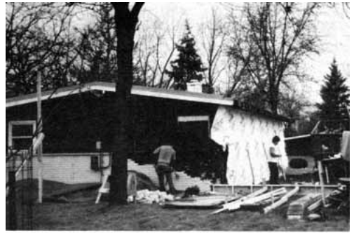
Figure 2. With the carport removed, the authors' crew prepares to pour a new slab for the family and dining rooms.
