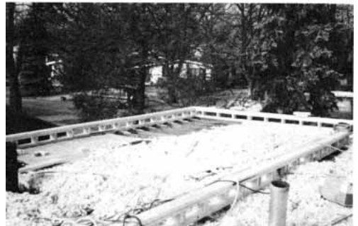
Figure 3. A 9-inch-high 2x6 wall separates the top of the ceiling joists from the bottom of the new second-floor joists, making space for plumbing and ductwork.
