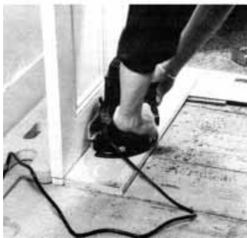
Figure 3. Because the floor slopes away from the door opening, the author had to support the saw on a piece of plywood to undercut the door. The plywood is blocked up to match the slope of the opening, so the cut will be parallel to the floor when the door is closed.
