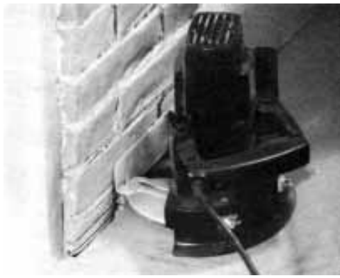
Figure 4. With a carborundum masonry blade, the Super Saw can undercut brick, block, stone walls, hearths, and chimneys. Here, an exposed brick pier is undercut to allow \frac{3}{4} -inch maple flooring to slip underneath it, allowing the floor to expand and contract without opening up an unsightly gap.
