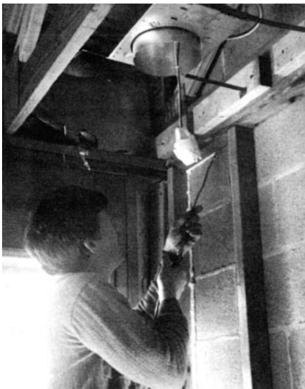
A house doctor seals off thermal bypasses by applying foam sealant between wood framing and a masonry party wall.
