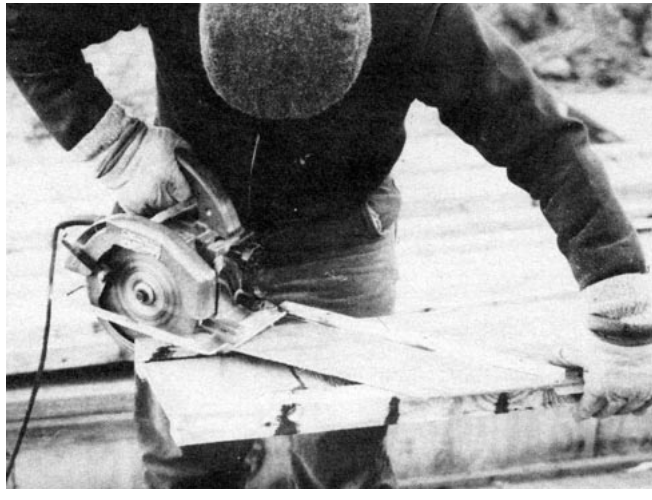
Figure 1. Hoch came up with this jig (top) to simplify marking and cutting I-beams. For plumb and cheek cuts, he holds the jig as you would use a Speed Square for crosscutting (above).
