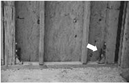
Figure 4. Two types of metal hold-downs are common in shear wall construction. Right-angle plates (top) bolt onto threaded foundation anchors and attach to 4x4 posts in the wall. Hold-down straps (bottom) are embedded in the concrete foundation and nailed to 4x4s through the sheathing.
