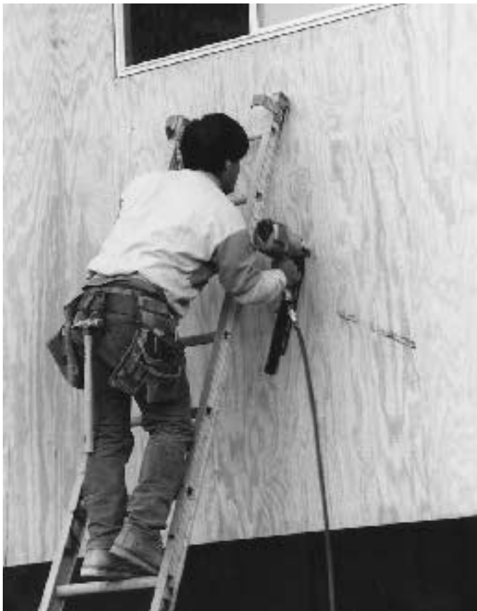
A carpenter in Mountain View, Calif., nails off a plywood shear wall with a pneumatic nailer.
