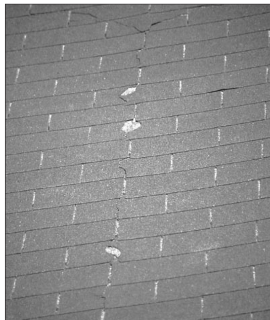
Figure 2. Fiberglass shingles that fail early usually crack, either vertically up the roof over many courses of shingles, or horizontally and diagonally across tabs.
