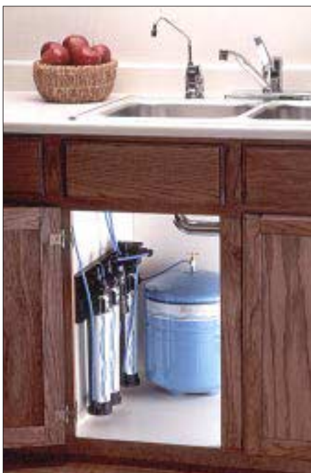
Figure 2. Point-of-use filtration is more common and less costly than central systems. This undersink reverse osmosis system from Culligan can deliver 1/2 gallon per hour and costs from $500 to $800 installed.
