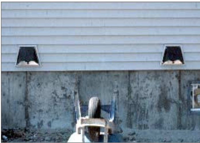
Figure 5. To prevent “short circuits,” the author separates intake and exhaust hoods by 4 to 6 feet. He also keeps them at least a foot above grade to prevent snow infiltration.
