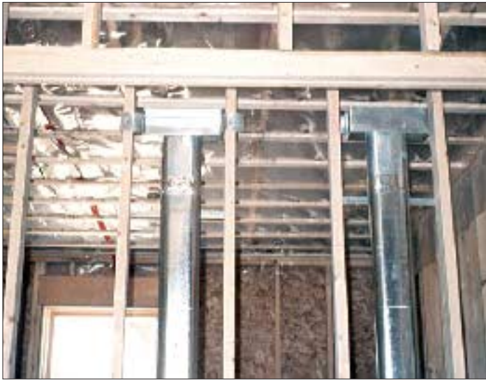
Figure 4. Placing supply and exhaust grilles high on the walls reduces drafts and helps cooler incoming air mix with the house air. For routing through stud bays, the author prefers oval ductwork because it is less expensive and easier to install than rectangular.
