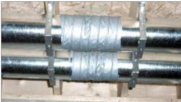
Figure 6. Interrupting a rigid duct run with a canvas connector helps keep HRV noise out of the ductwork.
