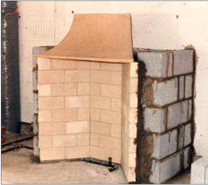
◀ Figure 3. The curved throat sits in refractory mortar at the top of a Rumford firebox built with ordinary firebrick.
