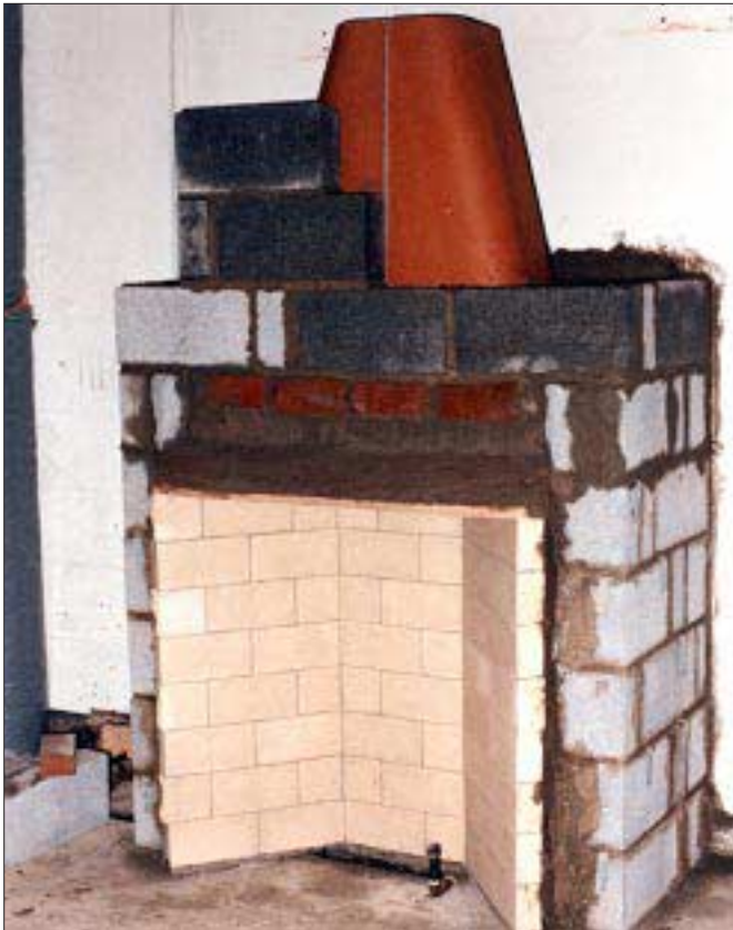
▶ Figure 5. The smoke chamber provides a transition to standard-size flue liner. It sits above the damper and is surrounded with ordinary bricks and mortar.
