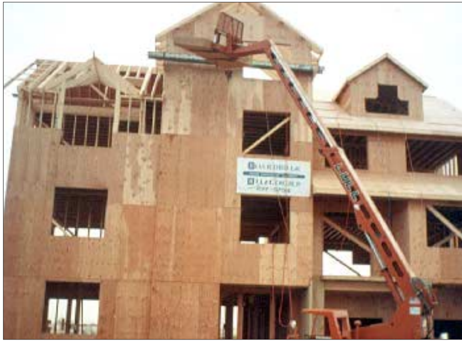
Figure 4. Because homes on pilings are typically quite tall, highlifts are indispensable timesavers when it comes to moving materials.
