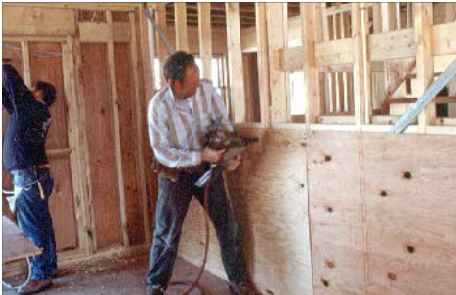
Figure 3. Bolted two-by X-bracing (top) and interior shear walls (above) help stiffen houses built on pilings. Both details must be engineered.
