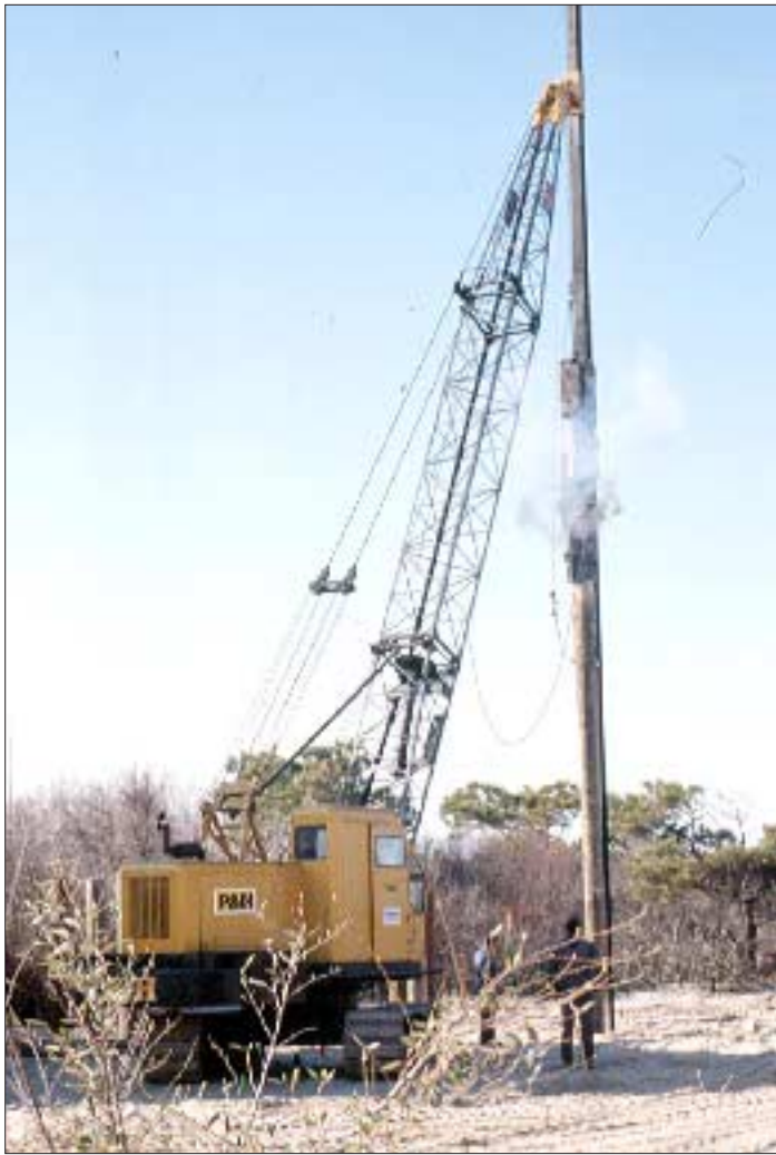
Figure 1. By counting the number of blows required to drive the piling a given distance, the builder can determine the pile's bearing capacity. A driving log is usually kept to show the inspector.
