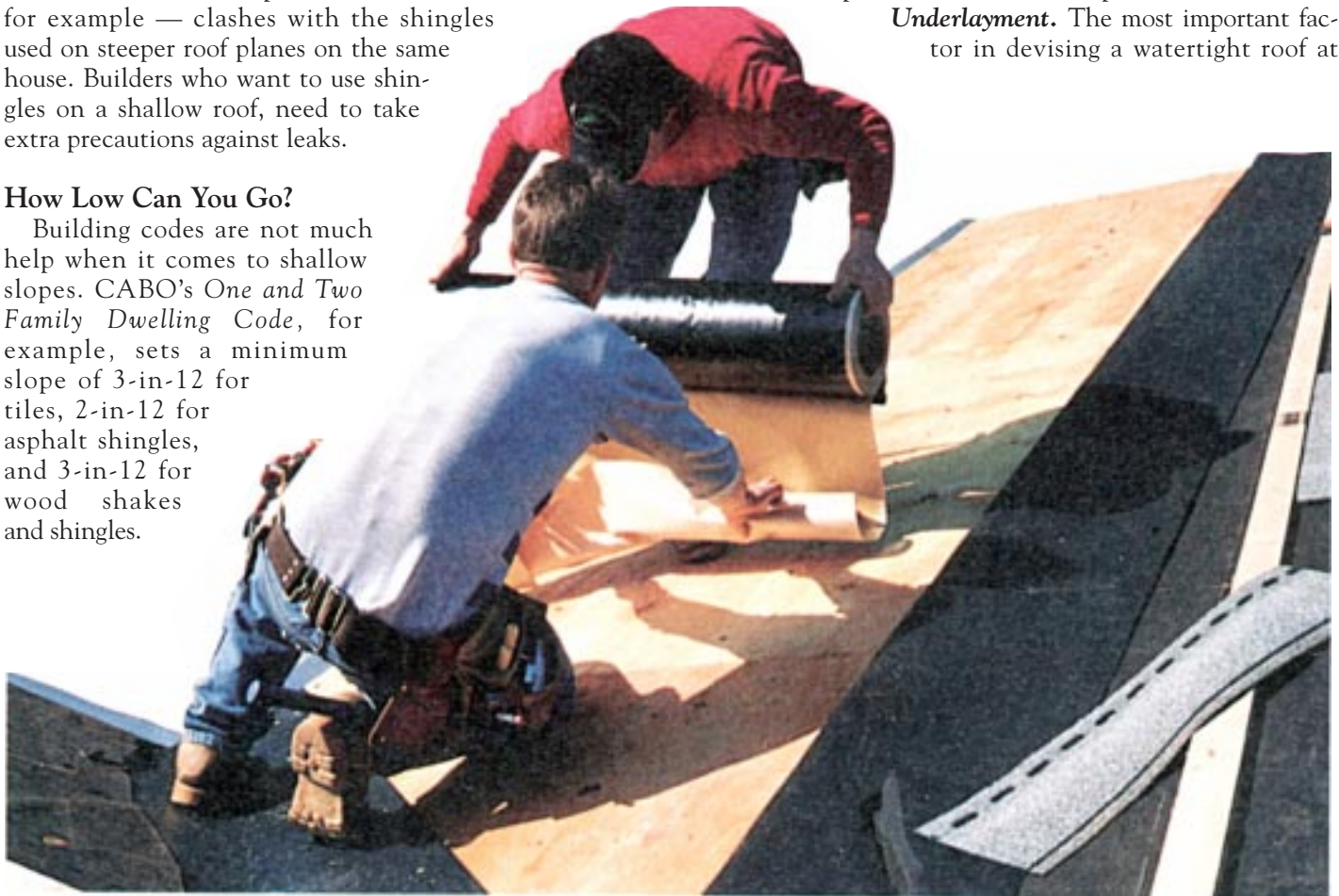
Workers place self-adhering bituminous membrane at the edge of a shallow-pitched roof. The membrane is installed by unrolling it across the roof while peeling off the backing paper. The job requires at least two sets of hands — one to hold the roll and another to smooth out the wrinkles.
