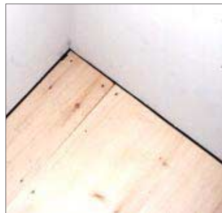
Figure 2. To allow for expansion, leave a \frac{3}{8} -inch gap between the flooring and the walls.
