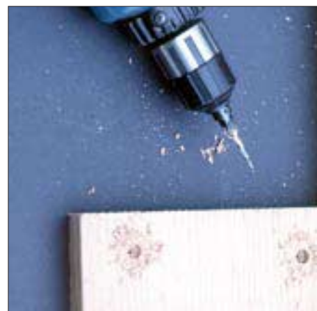
Figure 1. If you screw and plug a wide pine floor, you won't have to lay floor boards perpendicular to joists or align butt joints over joists. An adequately sized subfloor (at least \frac{5}{8} -inch plywood) will give the screw plenty of material to grab.
