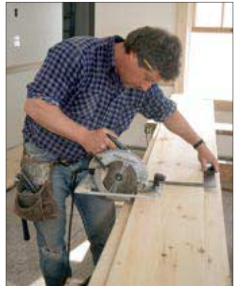
Figure 4. With extra wide boards, butt joints have to be cut precisely. For best results when you don't have access to a sliding crosscut saw, use a framing square, as shown, or a large Speedsquare, to guide the cross cut.
