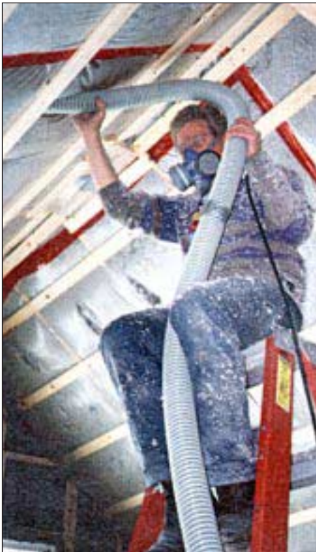
Figure 3. Here, dry cellulose is blown into a cathedral ceiling with a wet-spray blower. Wet-spray blowers can exert more pressure than conventional blowers used for dry cellulose. In this case, strapping has been installed to prevent the vapor barrier from bulging or breaking.
