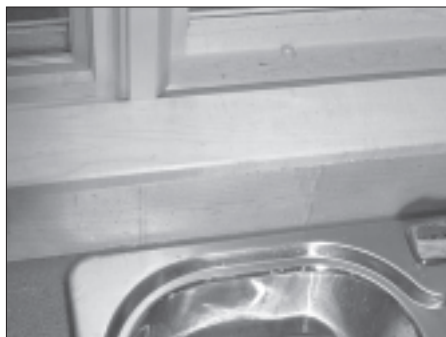
Avoid using wood backsplashes in very wet areas. This maple backsplash is still new, but it will deteriorate quickly from constant exposure to moisture.
