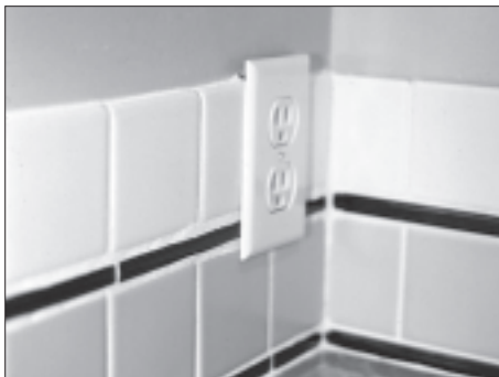
This electrical outlet interrupts the tile accent strip and protrudes beyond the top of the backsplash. The outlet should have been placed higher up on the wall.
