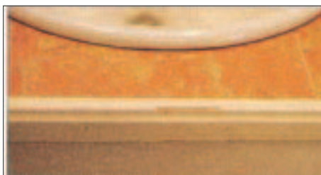
Figure 2. Painted wood edgings tend to break down quickly in damp environments, as happened with this three-month-old vanity. The best finish for wood edging is a good polyurethane.
