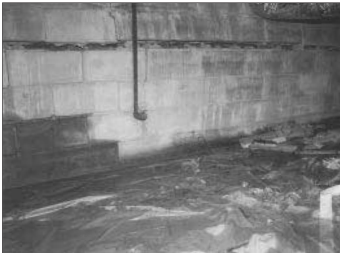
Figure 1. Horizontal cracks are common in unreinforced block foundation walls. Though they look threatening, such cracks move slowly and can often be repaired with simple measures.
