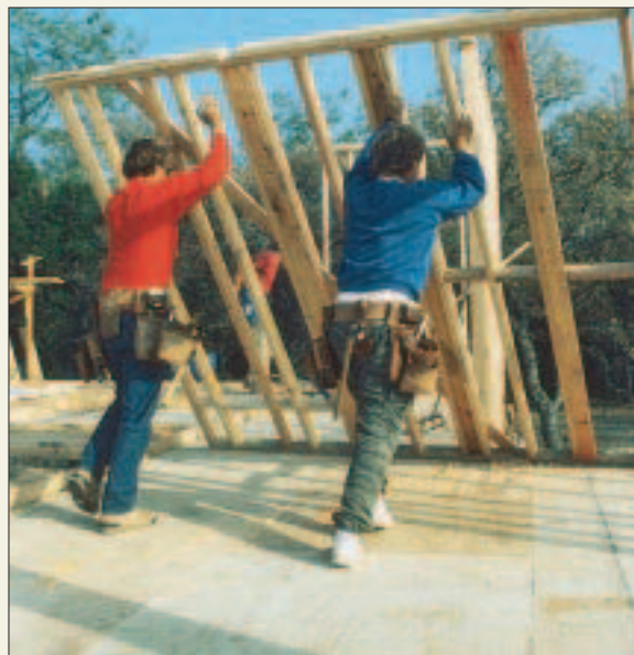
Heavy lifts call for extra care. Break the lift into stages and make sure you have enough manpower.
