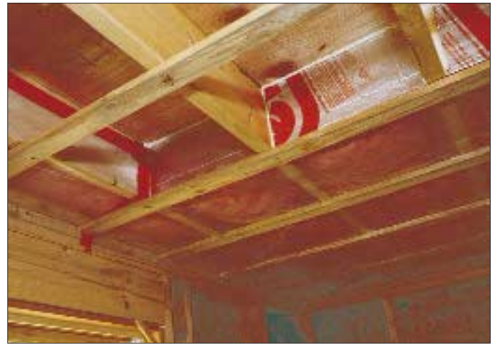
Figure 3. In new construction, rigid foam can easily provide an air block below an upper-story knee wall. Gaps are sealed with spray foam and the ceiling air/vapor barrier taped to the foil face of the foam board.
