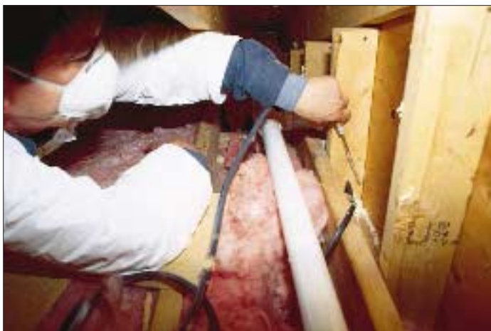
Figure 7. It's much easier to seal balloon-framed stud bays during framing than to have to do it later. Here, a weatherization worker foams a cardboard baffle into place where a gable-end stud bay passes into the attic.
