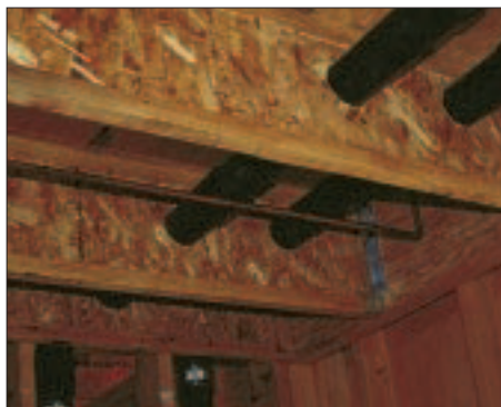
Figure 2. These large holes are too close to the end bearing point, so they compromise the strength of the joists. Follow the I-joist manufacturer's hole charts to avoid problems.
