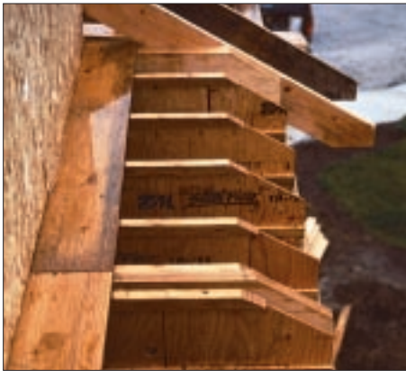
Figure 6. Beveling a joist beyond the inside of a bearing wall reduces its resistance to shear forces, which are greatest at the bearing. In this photo, the problem is made worse by the wall at the left, which rests on the joists with no bearing wall below.
