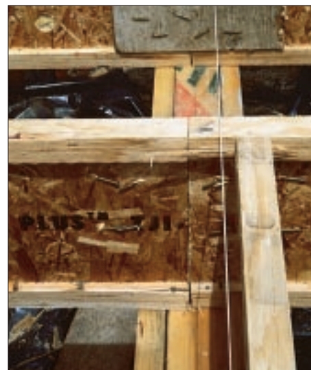
Figure 5. Avoid breaking an I-joist at midspan over a girder, as the builder did here. Crossing the girder with a continuous-span I-joist will yield a stiffer floor, and will not require full-depth blocking to resist rotation where the joists end on the girder. Note also the nail splitting the bottom flange, which reduces the joist's carrying capacity.
