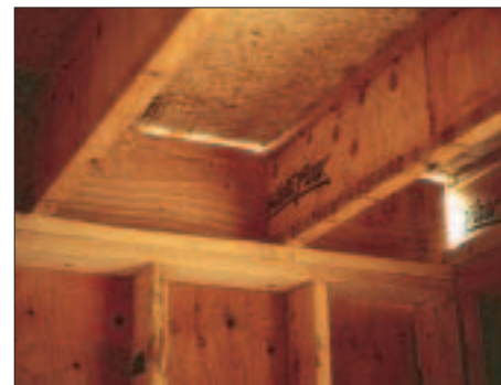
Figure 4. A 2-by rim joist is usually shallower than the I-joists; even if it's not, it will eventually shrink and leave a gap. This concentrates the structural load on the narrow joist webs, which aren't designed to support concentrated loads. Acceptable rim materials include I-joists, plywood strips, or an engineered rim material.
