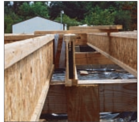
Figure 8. Where two or more I-joists serve as a girder, the web area should be filled in with blocking. The absence of blocking between the double joists in the photo means that the load at the joist hanger will be carried entirely by the I-joist it's attached to, instead of by the girder as a whole. The most likely result is a squeak or sag in the floor.
