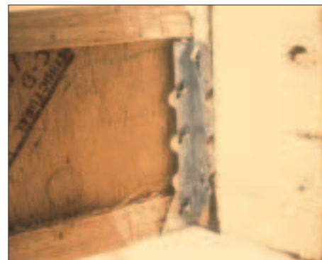
Figure 3. Because this joist hanger isn't tall enough to catch the I-joist's top flange, the joist may roll in the hanger. Note also that the builder has chiseled away the bottom flange to make it fit in the hanger, weakening the joist.
