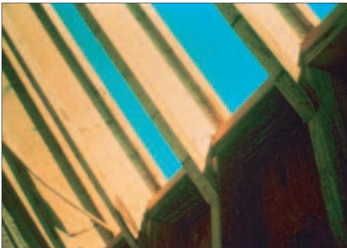
Figure 9. Notching a rafter over the inside edge of a wall leaves it bearing not on the heel, where it should, but on the toe. These rafters will split up the middle when loaded.
