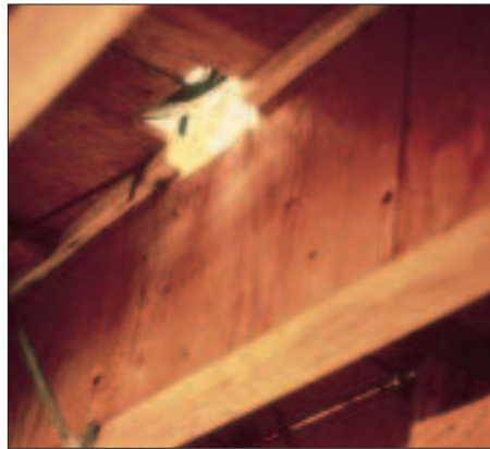
Figure 7. Notching the flange of an I-joist seriously weakens it; the closer the notch is to the middle of the span, the worse the problem. You can fix a notched joist by putting an additional joist next to it, or by removing the notched portion and supporting it with headers that span between the two adjacent joists.
