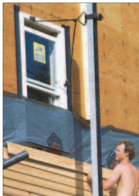
Figure 5. Because this carpenter has stretched the housewrap over the splines at the bottom of the window, wind-driven rain will be able to run down behind the housewrap onto the sheathing.
