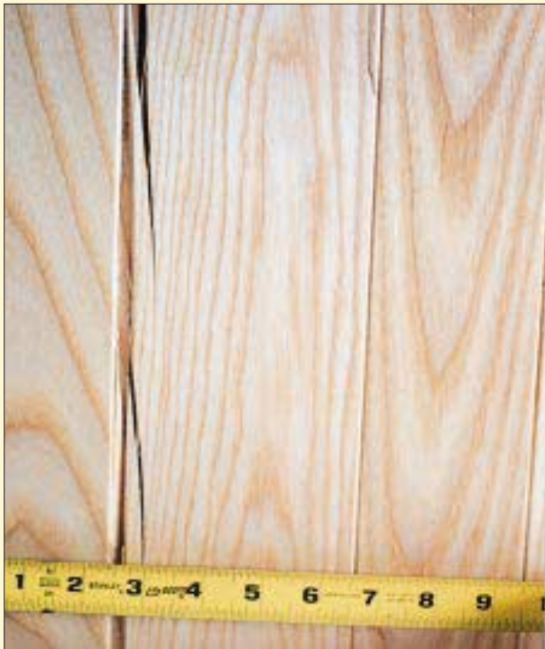
The edges of these ash floor boards were effectively glued together by the flooring finish. As the floor shrank in the winter, large gaps and splits occurred every six to seven courses.
