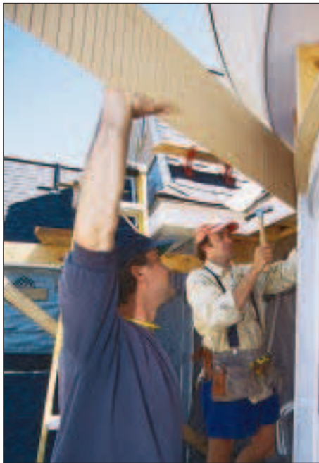
Figure 6. Exterior trim. Fascia, frieze, and exterior trim was kerfed on the back to make the bend.
