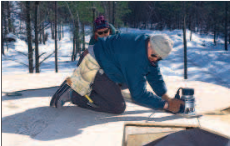
Figure 1. Router jig. A router on a pivot jig proved a necessity for making plates (top) and trimming subflooring (above).
