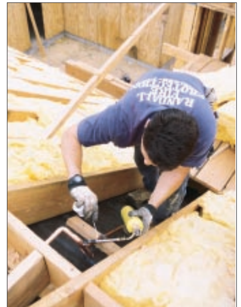
Figure 3. Residential sprinkler systems can be piped in CPVC, polybutylene, or copper. As polybutylene disappears from the U.S. market, cross-linked polyethylene is expected to take its place.
