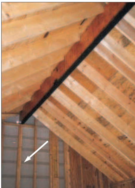
Figure 1. A double 2x4 post supports the structural ridge beam of this 16-foot-high cathedral ceiling. Is the post strong enough?
