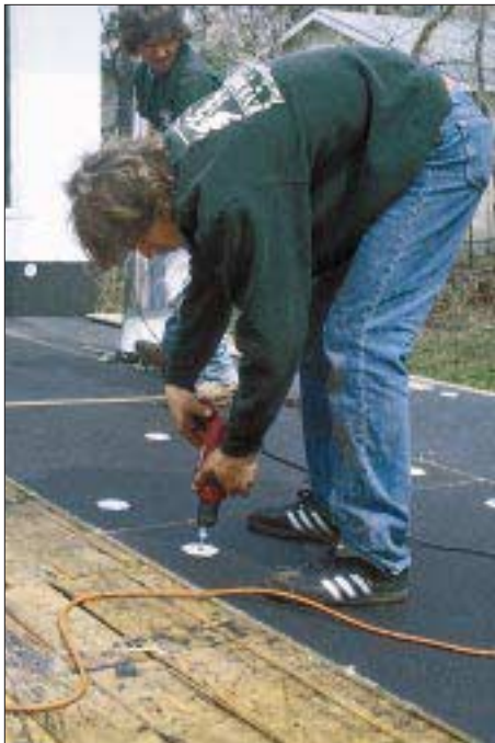
Figure 1. EPDM is installed over a special felt-covered insulation board. Screws and large metal fastener plates secure the insulation board to the roof deck.
