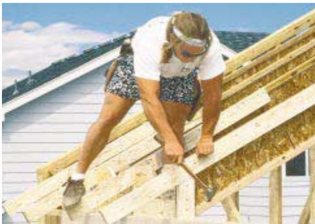
Figure 4. Many soffit profiles are possible with an I-joist roof system. Shown here are dimensional lumber rafter tails (left), a level soffit (middle), and an I-joist used as backing for fascia (bottom).
