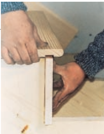
Figure 7. The author relies on careful joinery, finish screws, and construction adhesive to build squeakless stairs. The dado construction (photo inset) also hides any gap between the top of the riser and the tread.
