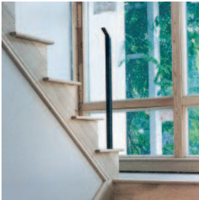
The tube runs through the tread down into the framing below, where it is securely lagged to solid framing.
