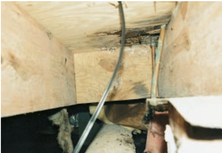
Figure 2. Localized plumbing leaks are easy to find. The repair usually involves simply replacing a small section of subfloor and occasionally beefing up a spongy joist.
