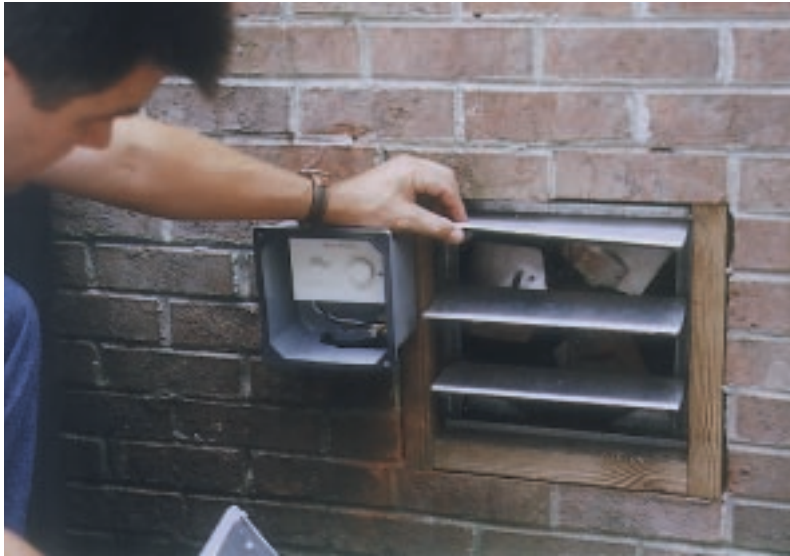
Figure 4. Rather than seal the crawlspace completely, the author uses a dehumidistat to measure crawlspace humidity and a humidistat to measure outside humidity. When the outside air is at least 10% drier than the inside air, these controls activate the fan to vent the crawlspace.
