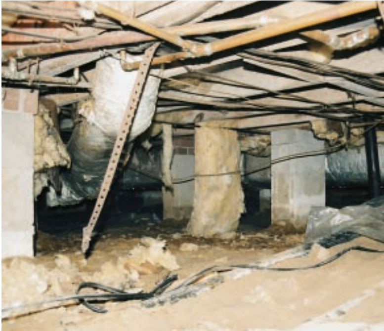
Figure 1. Crawlspace moisture problems often go undetected because homeowners are reluctant to scramble through the low headroom and the tangle of wires, pipes, and fallen insulation. Left unchecked, however, water from plumbing leaks, surface drainage, and a high water table can spur the growth of mold and mildew, and eventually lead to decay of sills and joists.
