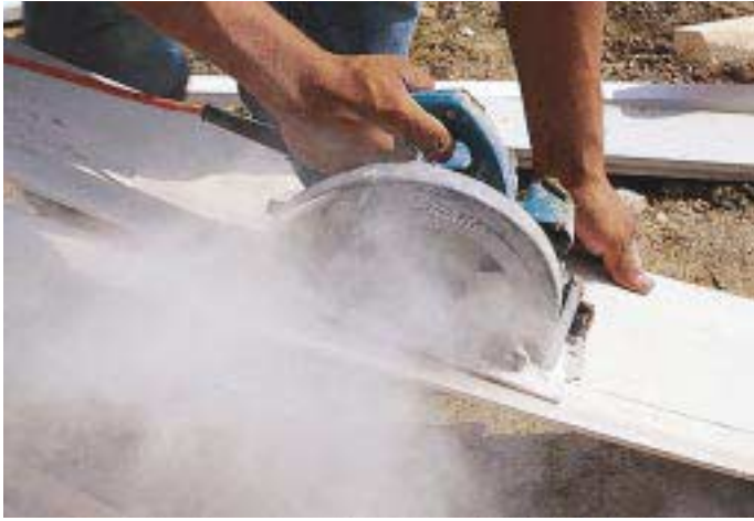
Figure 1. Most carpenters use diamond-tipped abrasive blades to cut fiber-cement, which is hard on saws and produces serious clouds of dust. Toothed blades cut faster and produce less dust, but the carbide tips dull fairly quickly.
