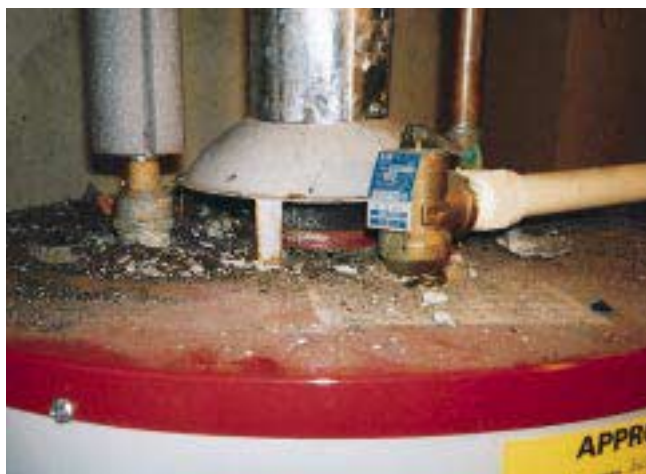
The top of this water heater shows evidence of flue gas spillage — the rust, paint discoloration, and debris are all clues to a backdrafting problem. A CO detector would give more immediate warning of the same problem.
