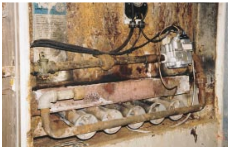
Some backdrafting problems leave obvious markers, such as the rust and corrosion inside this furnace burner compartment.
