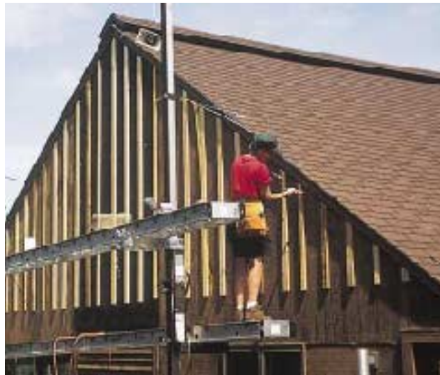
Figure 2. When re-siding the building, the author created a rain screen using vertical 1x3 furring strips 12 inches on-center. The resulting air space reduces heat buildup, and the equalized pressure on both sides of the siding prevents moisture from reaching the sheathing. The air space also permits any moisture that does accumulate behind the siding to drain freely.
