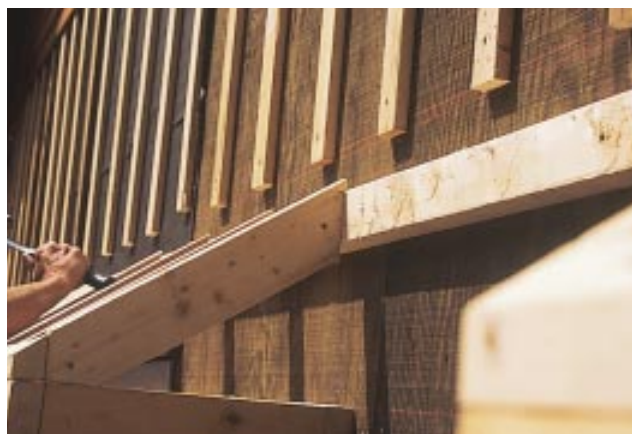
Figure 3. To protect both the windows below and the exterior shades, a shallow shed roof was built between eaves across the full width of the gable. The rafter tops were fastened high against a chamfered ledger to allow air entering through the soffit to flow into furring bays.
