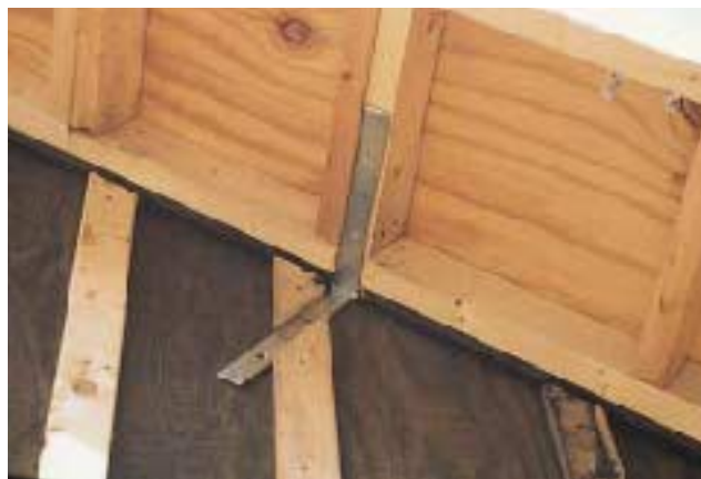
Figure 4. Because lack of an overhang contributed to the siding failure, the final step was to extend the rakes, which were supported at the bottom and midpoint with heavy steel angle brackets.
