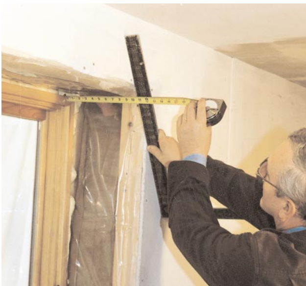
Figure 2. The secret to a precise final installation is careful measuring. The author checks both walls and window units for plumb, and uses a framing square and tape measure to check jamb depth at the corners.
