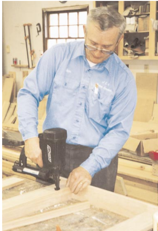
Figure 6. A Paslode Impulse finish nailer is the gun of choice for attaching the casing frames to the extension jamb boxes. The author finds that this airless nailer sets the nails better than pneumatic nailers. He also uses it on site for final installation of the units, avoiding the hassles of compressor and hoses.
