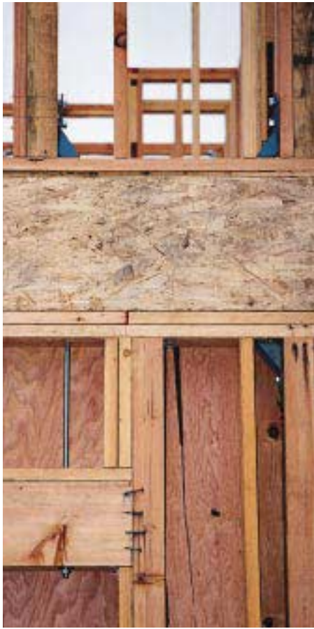
Figure 5. The window opening at the bottom left of the photo was enlarged, pushing the first-story hold-down post out of line with the second-story post. In a quake, the uplift forces will likely rip the long threaded rod through the header or pull the header out of position.
