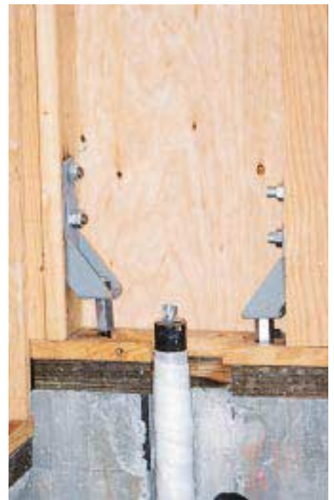
Figure 4. This shear wall is not long enough (plate length) to meet code, and the plate has been so badly mangled by the hvac sub that its lateral strength is compromised.
