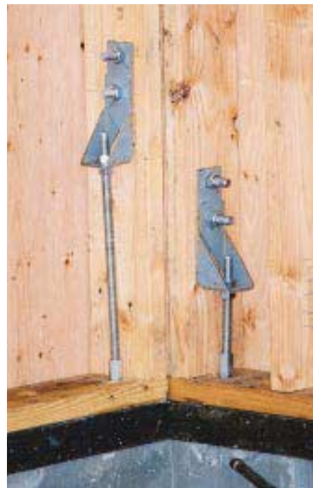
Figure 3. It's a mistake to attach two hold-downs to a single post. The two shear walls meeting at this corner should have been properly connected with nails, and one correctly sized hold-down attached.
