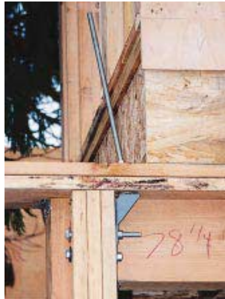
Figure 6. A triple-2x4 post makes it difficult for the carpenter to know where to place the perimeter nailing. The author recommends nailing off all three studs with the edge nailing schedule.
