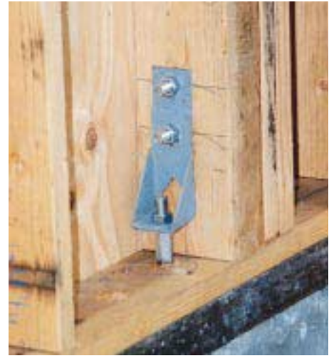
Figure 2. Assuming the anchor bolt is properly embedded, this hold-down is correctly installed.
