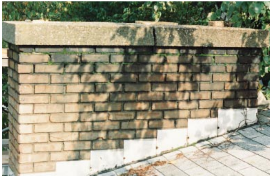
Figure 2. Excessive shrinking caused this crown to crack at the weakest point — the area where a flue penetrated the surface. Proper curing reduces the amount of shrinkage, and reinforcing fibers added to the concrete crown mix add tensile strength.
