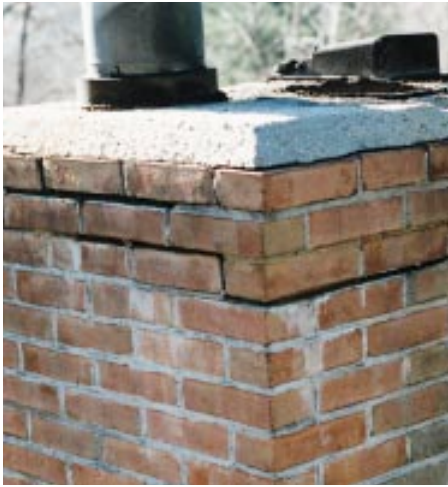
Figure 1. This chimney crown dried too quickly, causing the edges to curl and pull away from the masonry, allowing water to penetrate. This crown also bonded to the flue liners. When the liners expanded, they lifted the top of the chimney, causing the top three courses of brick to crack.
