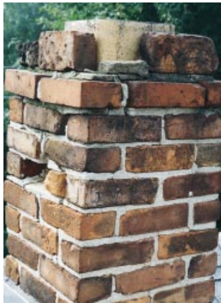
Figure 8. Older chimneys with deteriorated lime-and-sand mortar must be torn down to the roofline and rebuilt.
