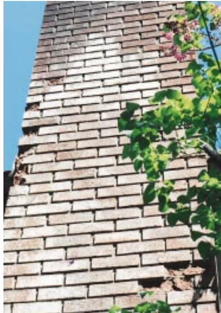
Figure 7. The decorative, deeply raked joints in this chimney allowed water to pool and soak into the brick. When the saturated brick was exposed to extended sub-freezing temperatures, the water froze and expanded, causing the brick to spall.
