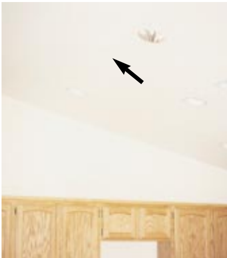
Figure 2. Residential sprinkler heads include pendant models (top) and recessed types (above) that are barely noticeable.
