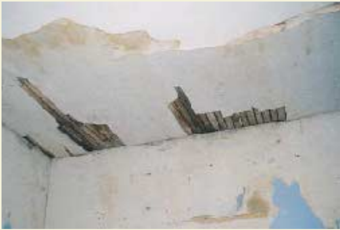
Plaster in this room was applied too thin and has stains from an earlier roof leak. New drywall is a simple fix.
