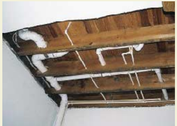
Sound floor framing is exposed where Dworin has roughed in new plumbing for the upstairs bath. A planned closet will support the joists he has drilled through.
