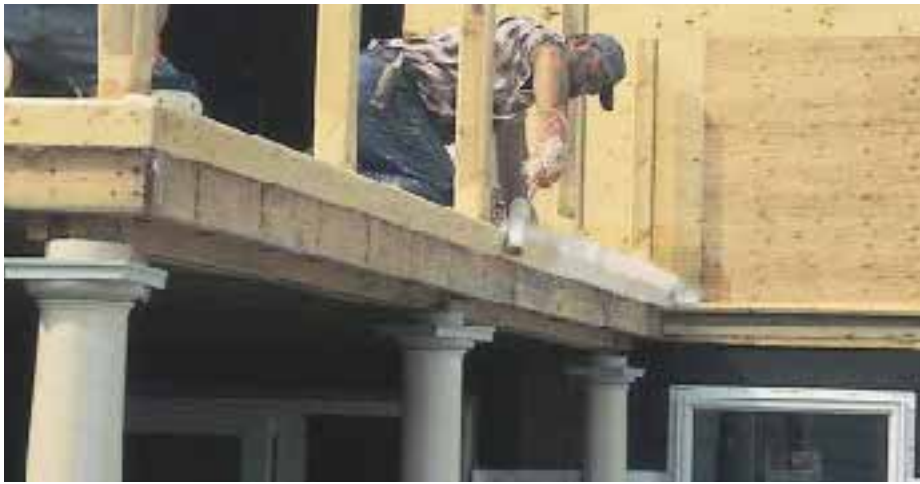
Figure 8. At the railing posts and perimeter drip edge, fiberglass mat flashing is bedded flush with the backcut bottom edge and wrapped up onto the deck surface, then coated and rolled.
