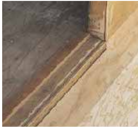
Figure 4. A 45-degree cant strip keeps water from ponding in the corners and prevents cracking in the fiberglass where it turns up the wall (top). At door sills, a narrow trim strip serves as a backstop for the fiberglass, which will create a seamless waterproof pan under the door (above).
