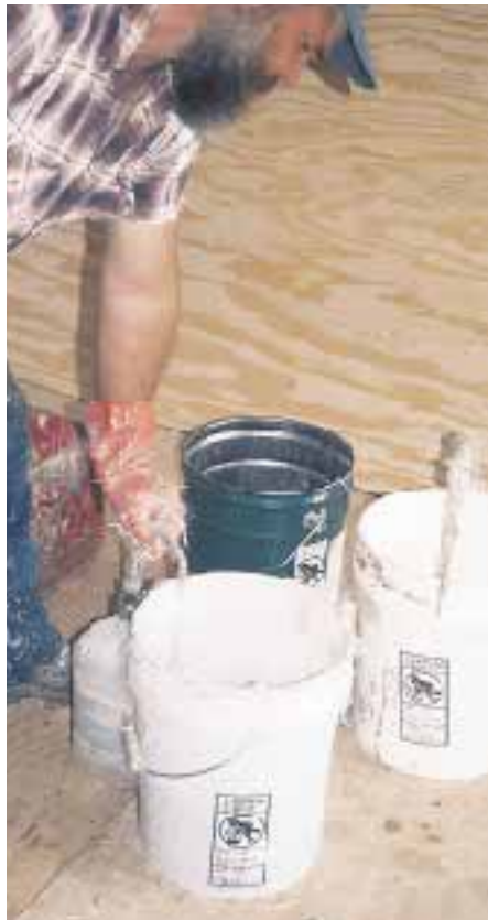
Figure 1. Fiberglass resin is mixed on site with a hardener (methyl ethyl ketone peroxide) in a ratio that can be varied to extend or shorten set time. The base coat is applied over plywood with reinforcing mesh at joints and penetrations, then finished with a gel coat.
