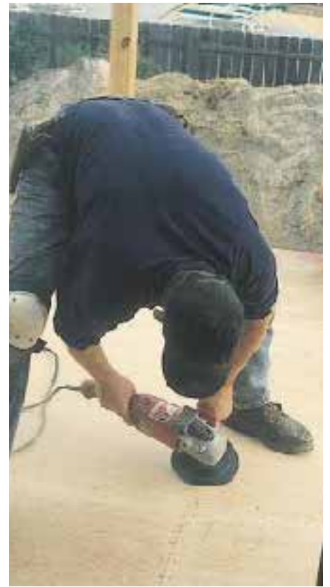
Figure 5. Before applying the fiberglass mat flashing, all edges — including the bottoms of railing posts, the edges of door openings, and all plywood joints — are knocked down with a coarse-disc grinder.
