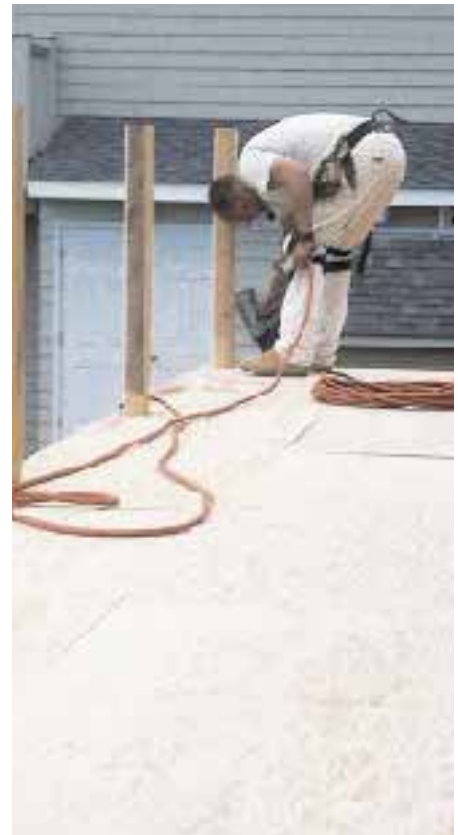
Figure 2. On the day the fiberglass will be applied, a clean, dry layer of 1/2 -inch AC plywood is laid over the base layer of 3/4 -inch T&G plywood. Joints are staggered and the sheets are fastened with 8d ring-shank nails.
