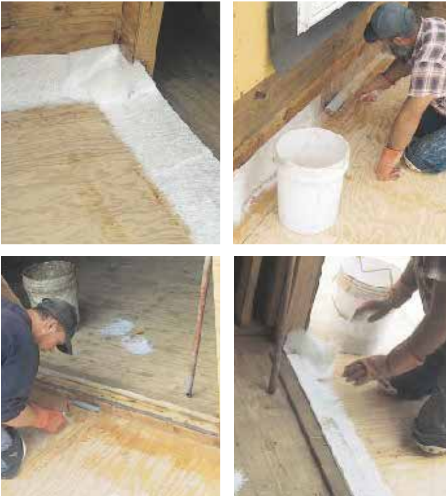
Figure 7. At cant strips, a band of fiberglass mat is pressed into a bedding coat of resin (top left), then coated with more resin (top right) and rolled with a small steel roller to force out any trapped air (above left). Door sills get the same treatment (above right).
