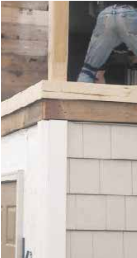
Figure 3. A 1x4 fastened to the rim joist will be wrapped with fiberglass to provide a clean termination at the deck perimeter. Fiberglass doesn't bond well at 90-degree corners, so the top outside edge of this trim piece is eased with a 1/2-inch round-over router bit. A 20-degree ripped undercut serves as a drip edge.
