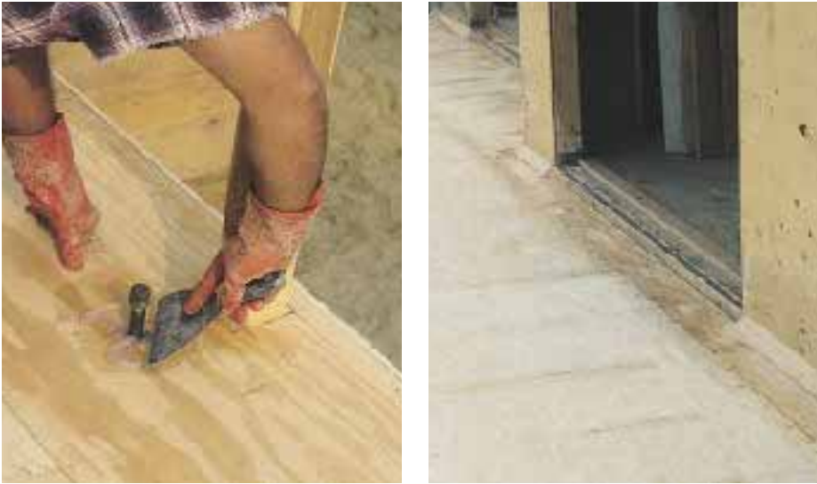
Figure 6. A site-mixed fiberglass and silica leveling compound is applied to all joints and nail heads, and is used to fill in gaps around posts and other penetrations (left) and at cant strips and door sills (right). When dry, any lumps and high spots are hand-sanded.
