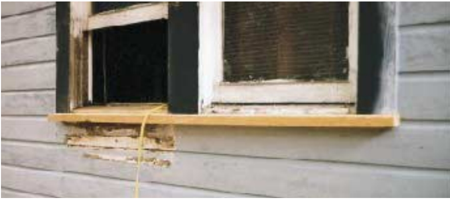
Figure 1. The author makes replacement sills from pressure-treated Southern pine. At 19 degrees, they're angled more steeply than the originals to shed water better.
