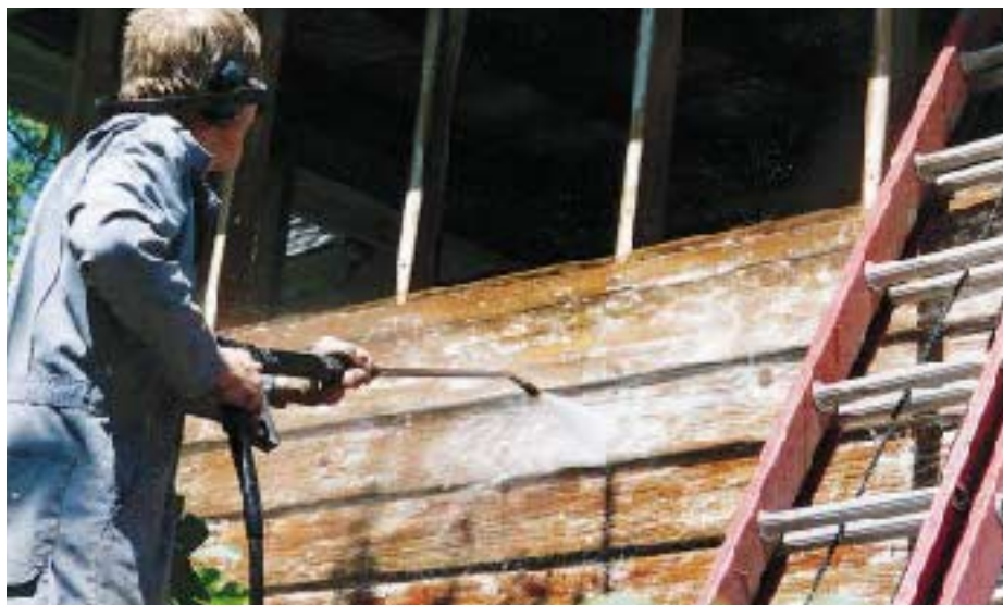
Figure 7. Pressure-washing stripped siding deep-cleans the pores of the wood. Note how the author "boxes out" an area of work, and the difference between the unwashed wood (top) and the washed wood (above).
