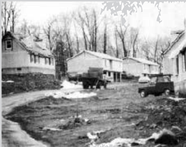
On-site work in this Connecticut modular development included pouring concrete foundations and finishing the siding and roof.
