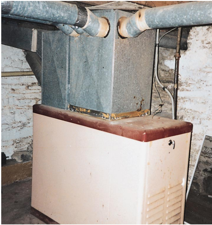
Figure 2. Because it was oversized, this 90,000 Btu furnace had to be replaced. The four 7-inch-diameter ducts carried only half the hot air the furnace was capable of producing, causing the heat exchanger to overheat and crack.
