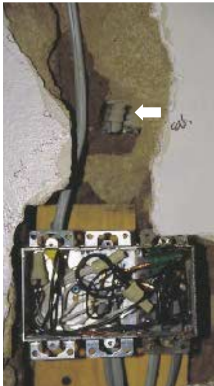
Figure 1. If you abandon existing work, make sure it is cut far enough back so it can't be reconnected, like the armored cable near the top of the photo.
