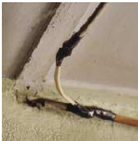
Figure 2. All splices must be in a box with an accessible cover plate. A splice must never be concealed in a wall cavity.
