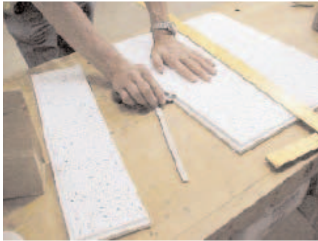
Figure 9. The surface of the rolling scaffold is a convenient surface for cutting tile. Cut edges of tegular tiles — sometimes called “shadow line” tiles — must be rabbeted as shown to fit the grid.
