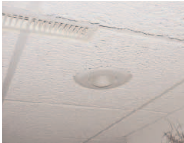
Figure 10. Recessing can lights and grills into the tile — leaving a reveal that matches that of the rabbeted edges — is a minor detail that results in a better-looking job.
